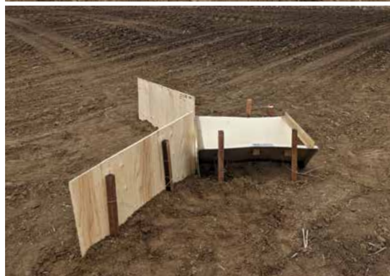
FIGURE 12. Example of H-flume installed at the exit point of the surface ditch from each basin.
