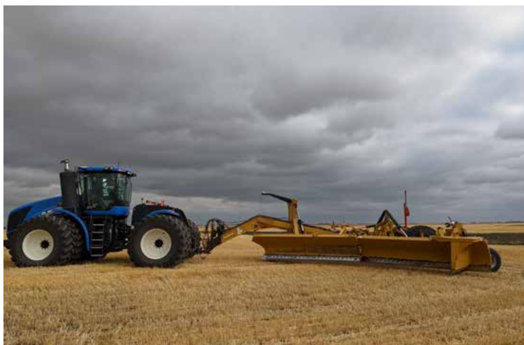
FIGURE 10. Pull dozer style plow used for construction of surface ditches to channel water from basins.
